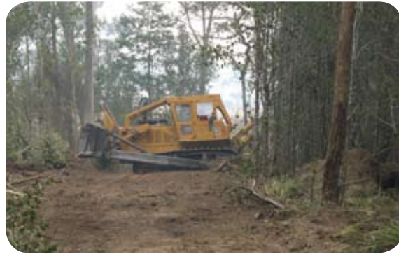
Earthmoving equipment is used during firefighting for construction of access roads and fire breaks. Photo courtesy of Paul Black, PWS.
