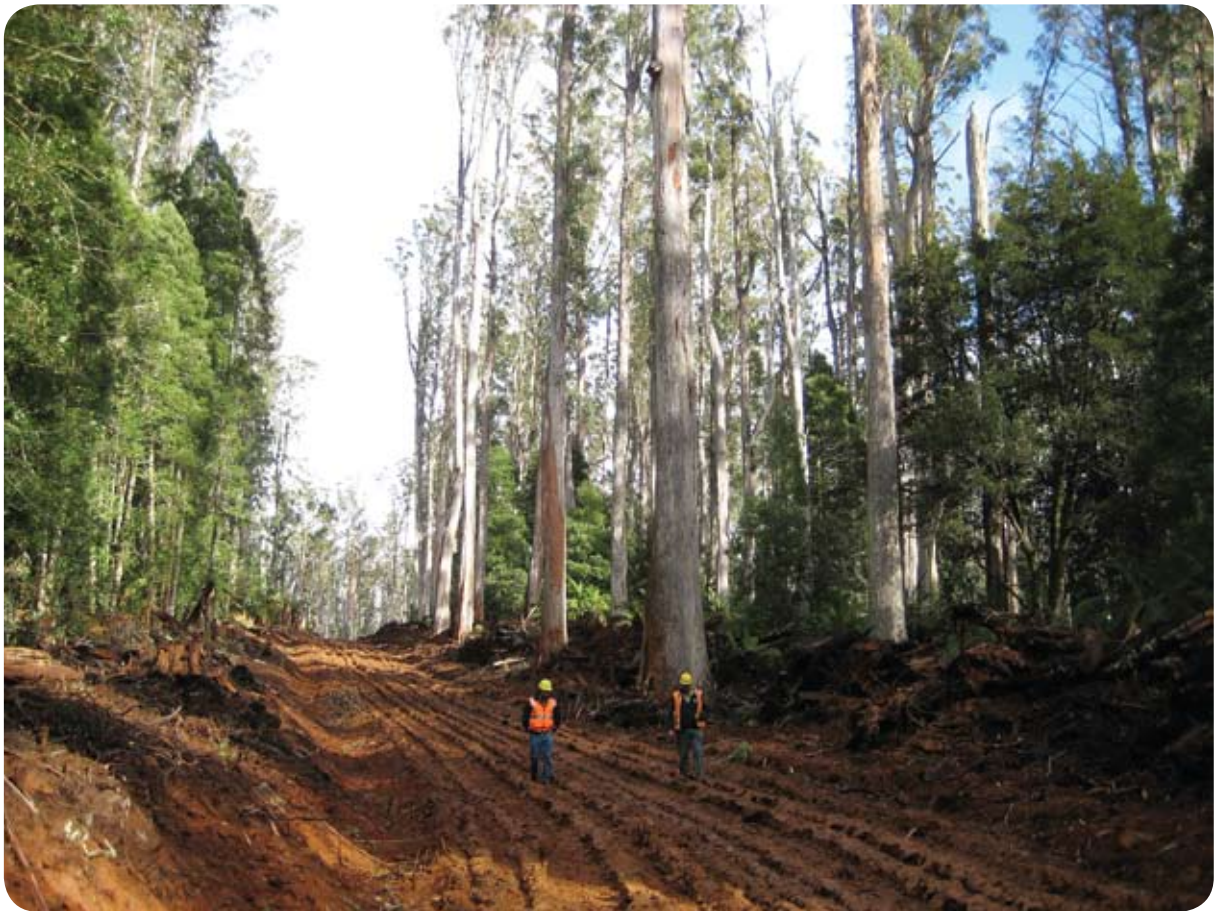
Constructing and maintaining dirt roads are a high risk for the spread of freshwater pests and diseases. Photo courtesy of Forestry Tasmania.
